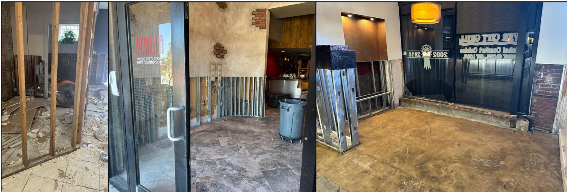
Figure 7: Interior and content damage of commercial buildings in Punta Gorda.
